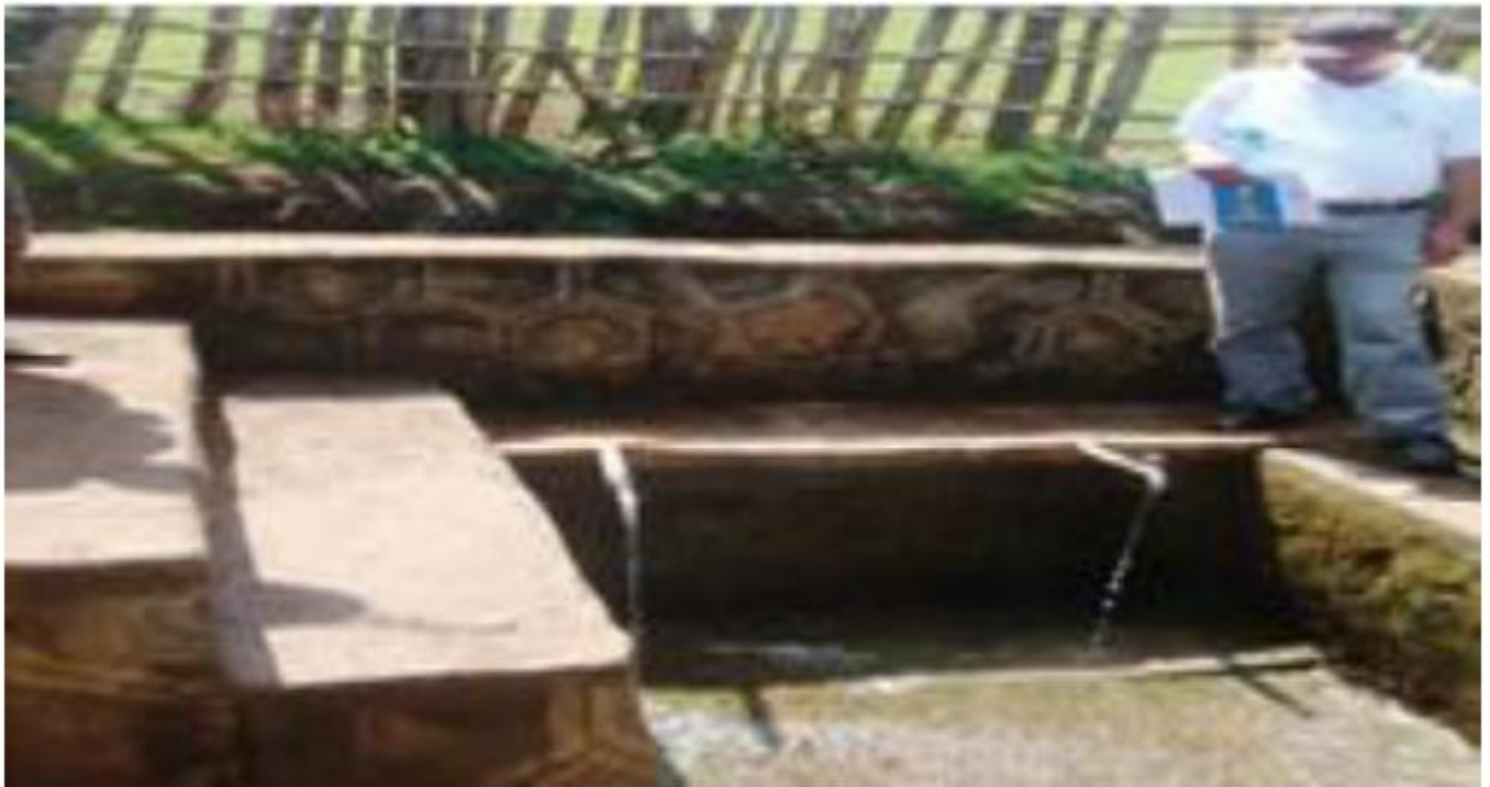
Figure 7.4: A protected spring. Note the concrete retention wall with two delivery pipes and the surrounding fence.
